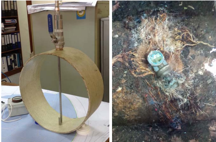
Figure 11 Typical large diameter tapping (Source: K Atkinson (1, 2)).
