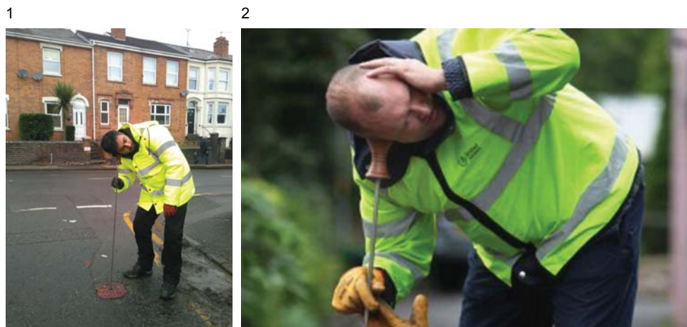
Figure 30 Photographs showing use of manual listening stick (Sources: K Atkinson (1), United Utilities (2)).
