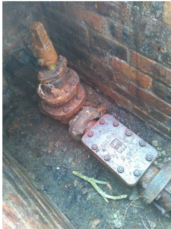
Figure 43 Typical pigging chamber (Source: K Atkinson).
