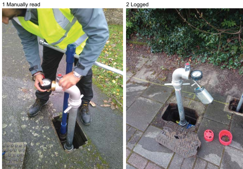
Figure 33 Photographs showing hydrant being used during a PZT (Source: K Atkinson (1, 2)).
