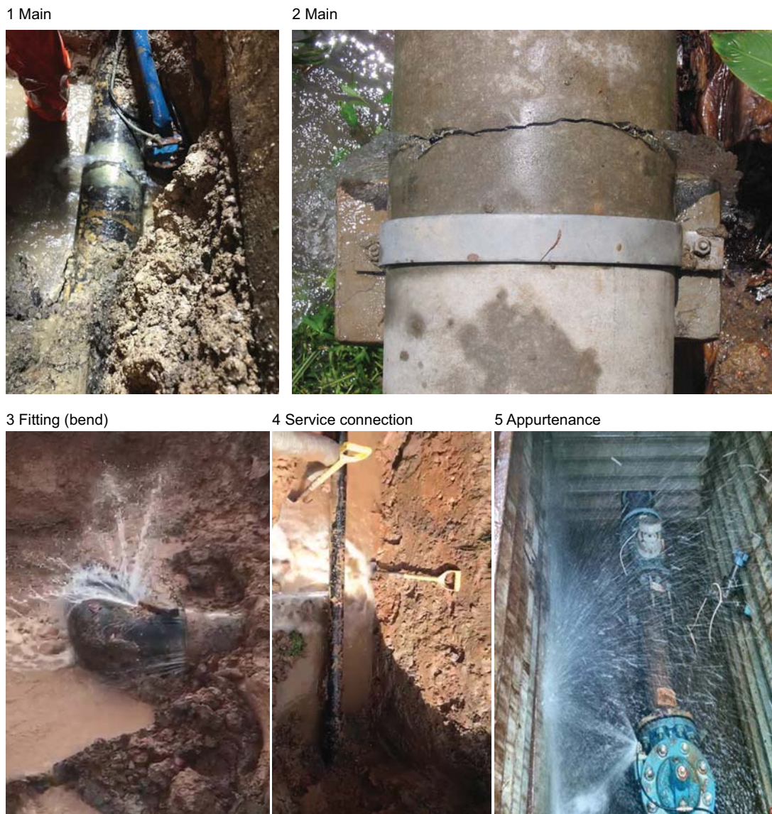
Figure 26 Typical leaks (Sources: Severn Trent Water (1, 3, 4, 5), K Atkinson (2)).
