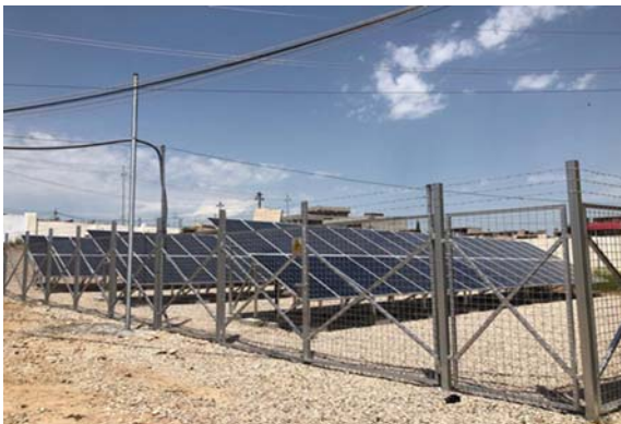
Figure 8.2 Solar-powered water project in Shekhan.
