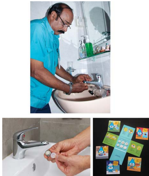
Figure 10.12 Example of installation of water efficient devices in homes (PUB Singapore, 2013).
