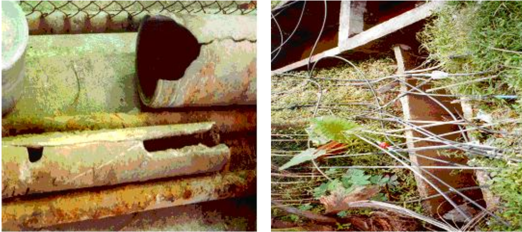
Figure 3. Photos of Burst Mains and Illegal Service Connections
