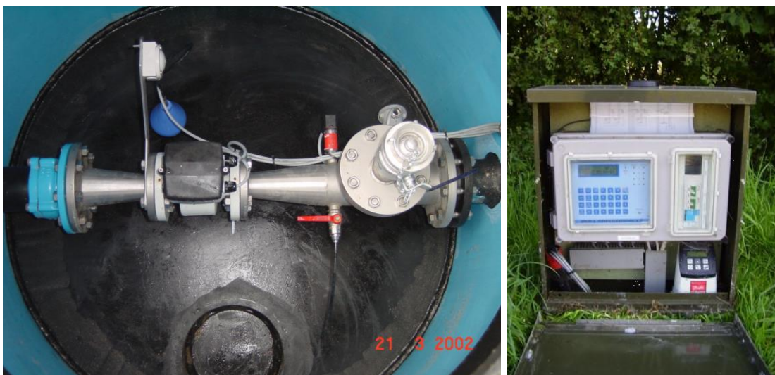
Figure 13 – District meter manhole (left) and installation cabinet for district meter.
