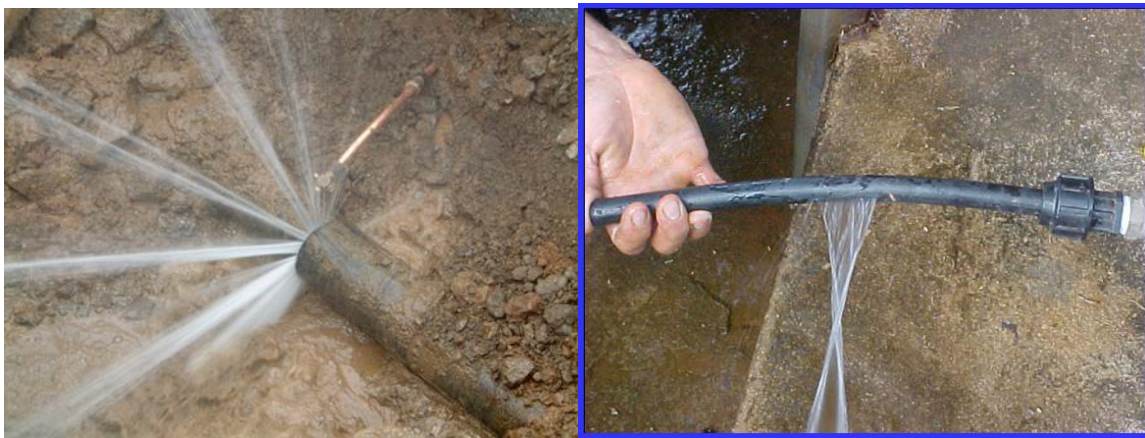
Fixed Area leaks – ring cracks, corrosion holes, blow-outs in rigid pipe materials. N1 = 0,5, Less sensitive to pressure changes
