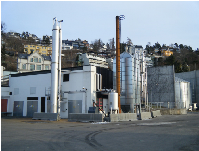
Figure 18.3 The biogas upgrading plant at Bekkelaget, Oslo (picture courtesy: Oslo Water and Wastewater Authority, Norway).
