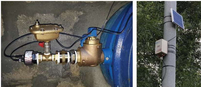
Figure 9.2 Solar-powered 3G data gateway on a nearby pole (right) and hydrophone sensor with external antenna and battery pack, plus automatic bleeding valve (left). (Source: Gutermann)
