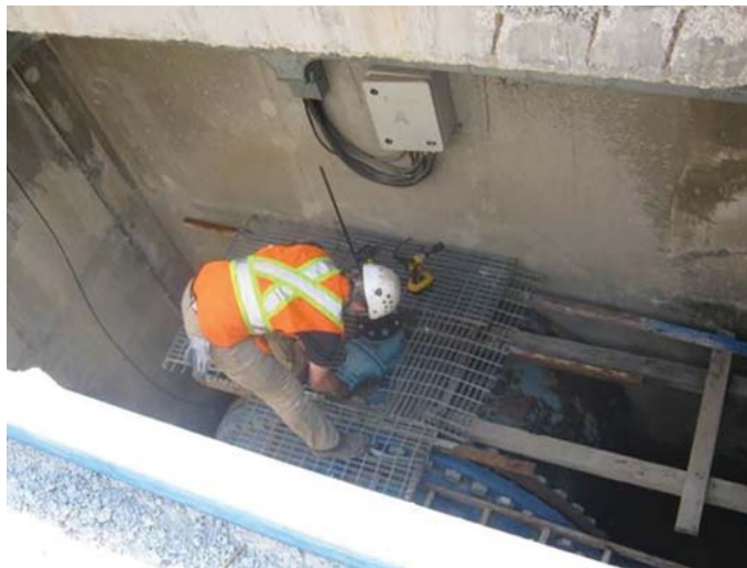
Figure 17.5.1 Leak located in excavation. (Source: Pure Technologies)
