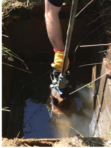
Figure 17.17.1 Enigma-hyQ logger installed on 500 mm PVC main via fire hydrant. (Source: Primayer)
