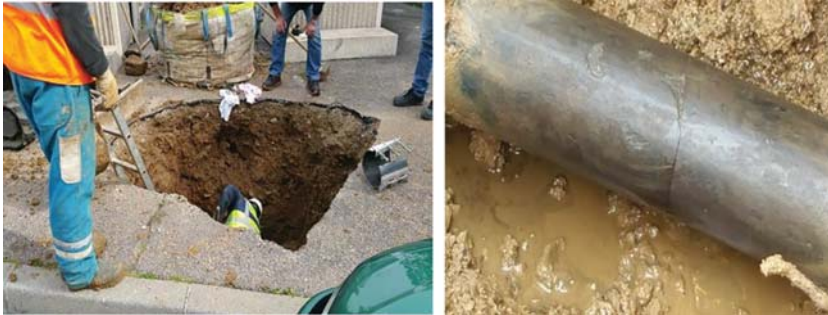
Figure 4.12 Excavation and leaking pipe exposed. (Source: Primayer)
