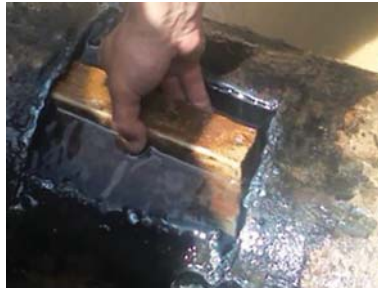
Figure 17.7.2 Length of wood located and removed from main. (Source: JD7 Ltd)
