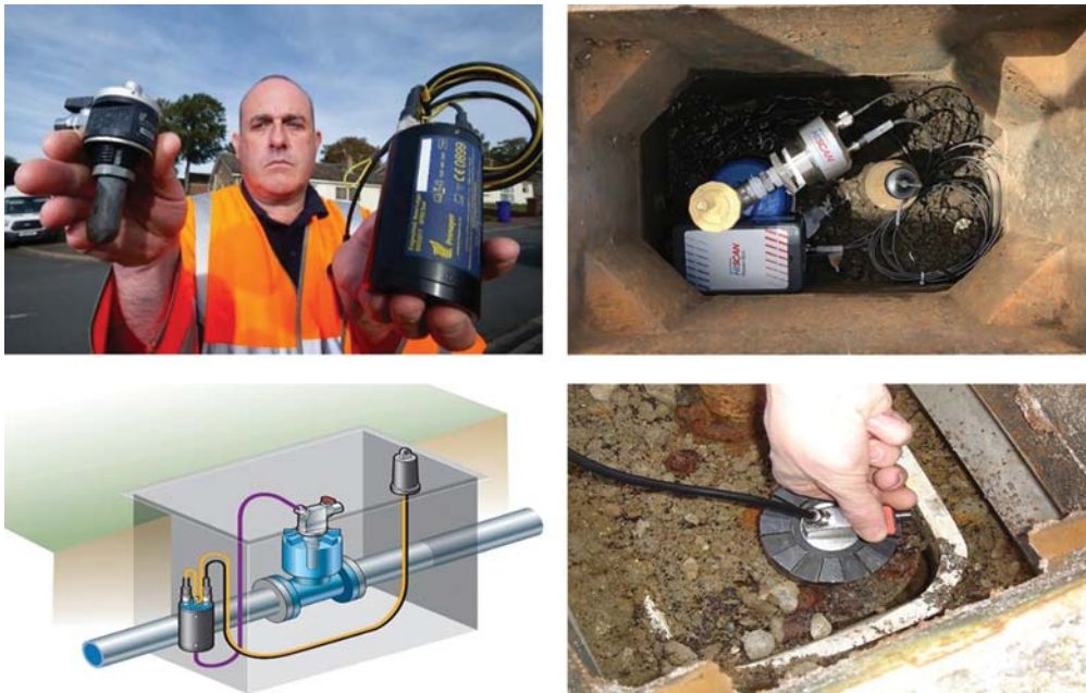
Figure 4.4 Example hydrophone installations. (Sources: Primayer (top left), Gutermann (top right) and Primayer (bottom))
