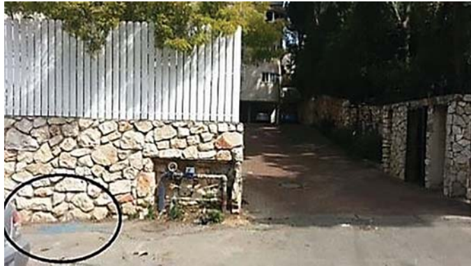
Figure 17.12.7 Leak position marked in blue by contractor. (Source: Gutermann)
