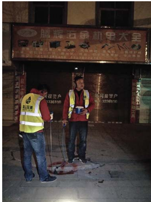
Figure 17.9.7 Leak point pin-pointing. (Source: Yunnan Kan Zheng Water Loss Control & Engineering Co., Ltd)
