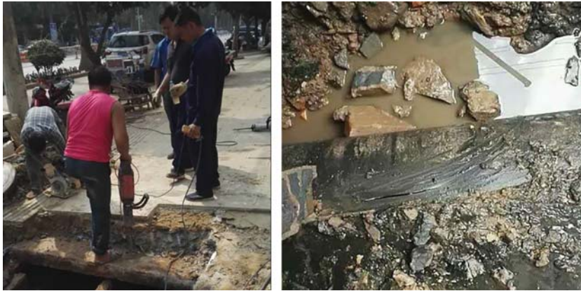
Figure 17.9.8 Leak point confirmation. (Source: Yunnan Kan Zheng Water Loss Control & Engineering Co., Ltd)
