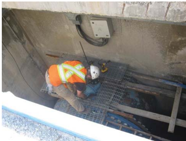
Figure 5.3 Leak located in excavation ( Source: Pure Technologies ).
