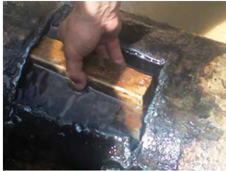
Figure 5.6 Length of wood located and removed from main (Source: JD7 Ltd).
