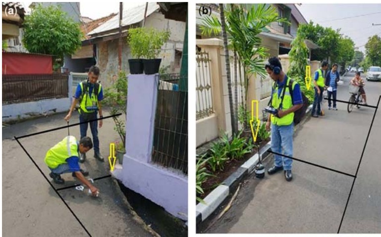
Figure 7.5 (a,b) Checking for leaks. Note: lines indicate the location of the pipework and the arrows indicate where the service pipe enters the property. (Source: Stuart Hamilton).
